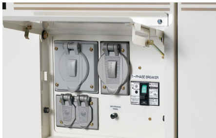
Convenient receptacles include 3-phase 480V, single-phase 120/240V and two 120V duplex receptacles.
